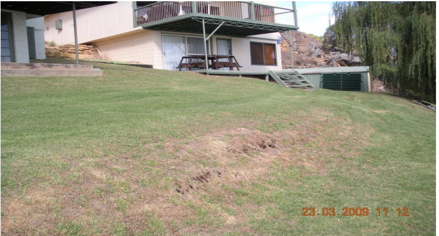
Cracks appearing away from the river
