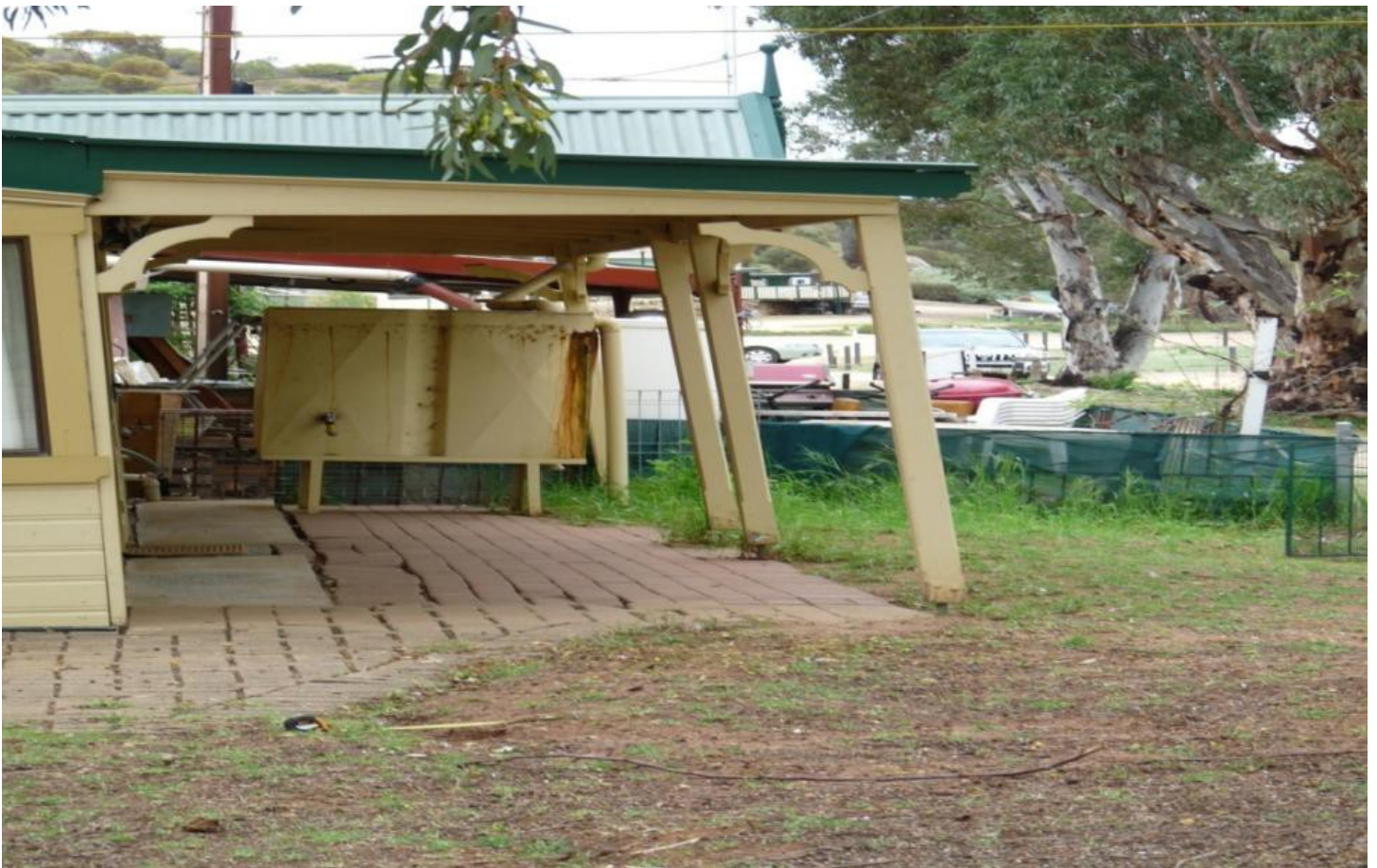
Damage caused by cracking and shifting soil
